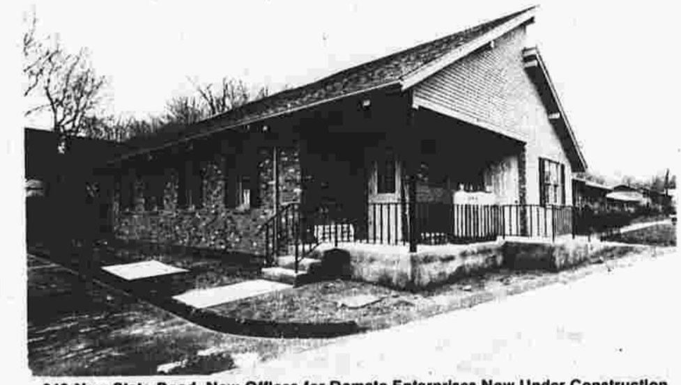
240 New State Road, New Offices for Damato Enterprises Now Under Construction (Sunny Brooke Village)
